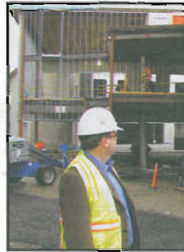
Scappoose Superintendent Paul Peterson checks in on construction of the new Petersen Elementary School.
